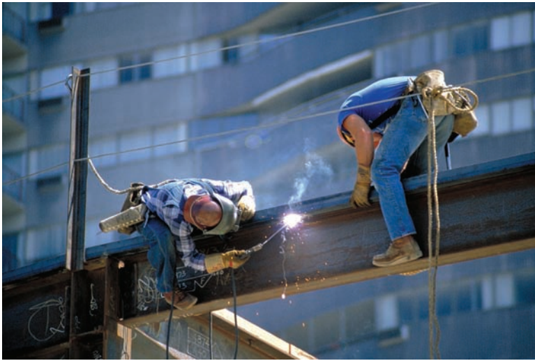
Fig. 1-11 Welders in the construction industries are called upon to weld in many unusual positions. Here, a welder and a helper are making an attachment to a building beam in the overhead position. The shielded metal arc welding process is being used and is being applied in the typical manual fashion. Note the safety gear and fall protection devices. © Vicki Silbert/PhotoEdit
